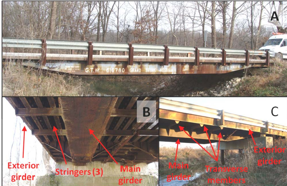
Figure 3.2: Typical RRFC, elevation view (A), longitudinal members from underneath (B), & transverse members from side (C)
