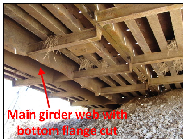
Figure 3.21: RRFC bridge with missing bottom flange
